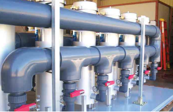
Custom skid mounted pre-plumbed cartridge filter system.
