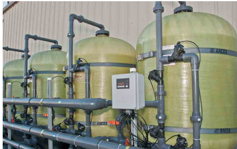
Parallel 48" x 72" Quad Carbon filter system with sequential backwash.
