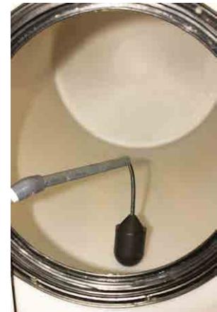
Pre Installed Float Switch
